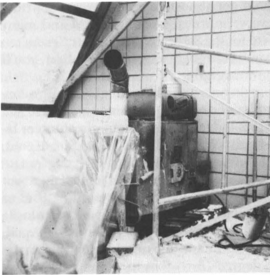
Kerosene-burning "salamanders" kept the drying concrete in the plastic enclosures from freezing during the construction of the stake center, winter of 1965-66.
